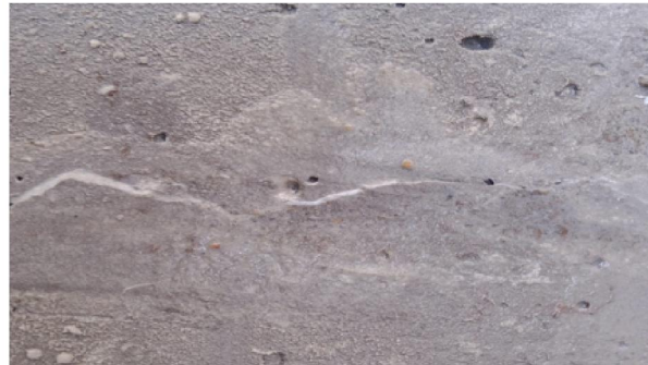
Fig 5: Healing of cracks on concrete surface
