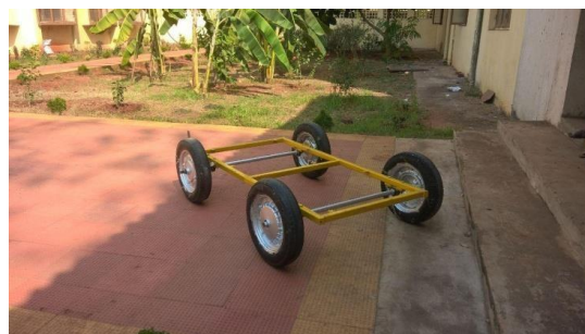
Fig 5.3.1 Frame of ms steel of 1.5 inch welded as a frame using arc welding
