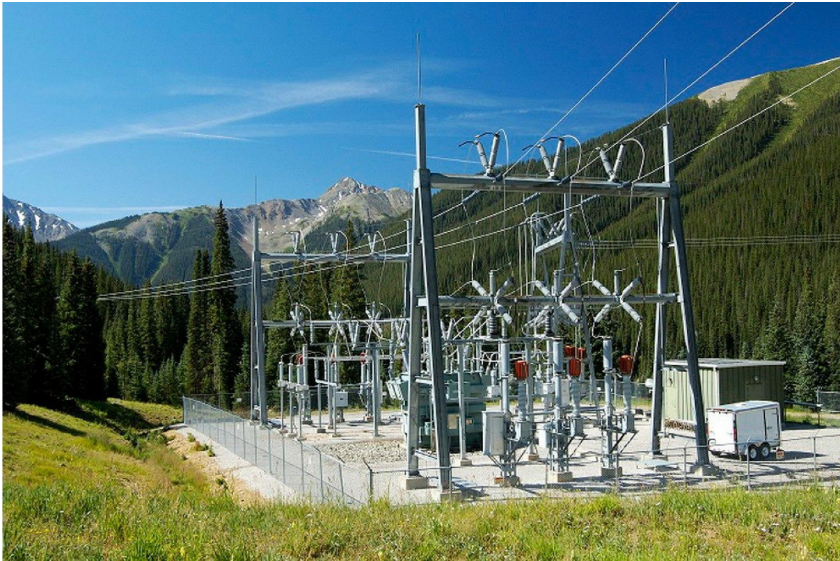
Fig 1.2: step down outdoor substation
