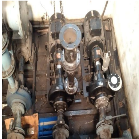
Fig 5: Three Phase Motor
