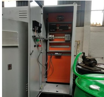
Fig 2: CCS control panel
