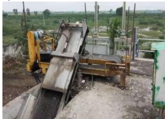
Fig 10: Screen Channel & Belt Conveyor
