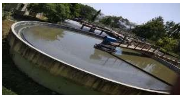
Fig 6: Secondary Settling Tank
