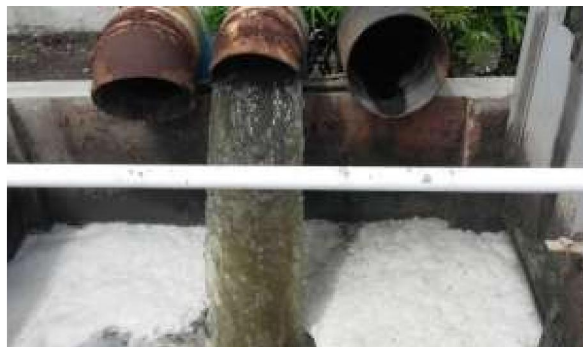
Fig 9: Plant Inlet Wastewater
