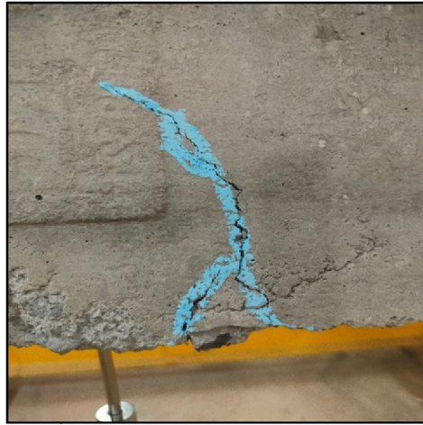
Fig 11: Single Crack Pattern in Concrete Beam
