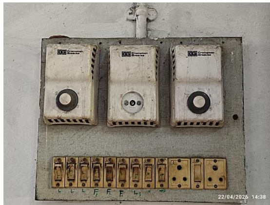
Regulators and switch board
