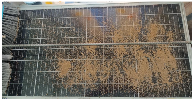
FIGURE IV SOLAR PANEL COVERED BY DUST AT 30%
