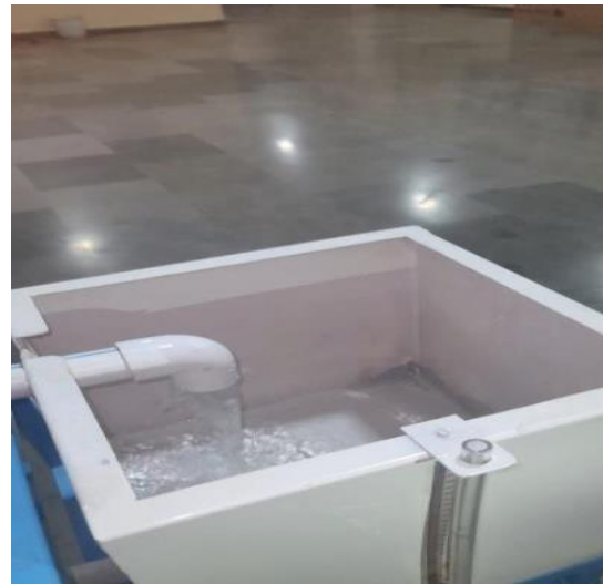
Fig 5.1 Water Tank & Manometer
