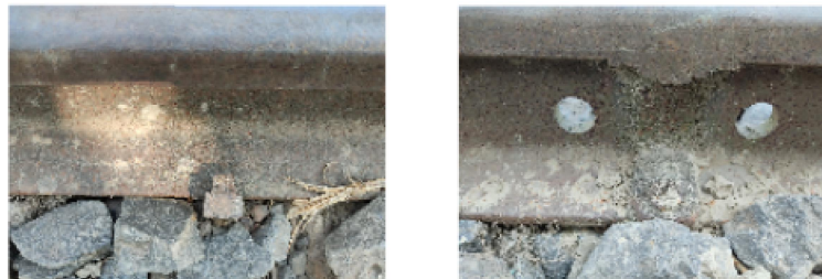
Figure 4: Defective Railway Links
