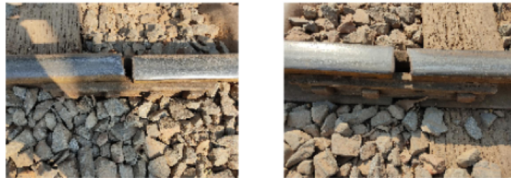
Figure 2: Defective railway tracks
