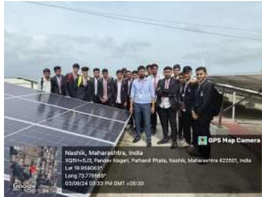
Fig.3: 200 KW Grid Tie System
