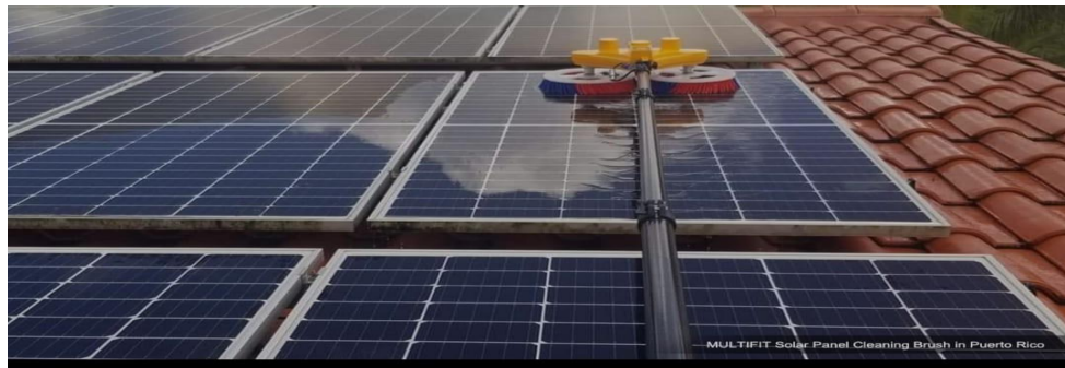
Figure 3.2:- Sun Brush full automatic cleaning over solar panels.
