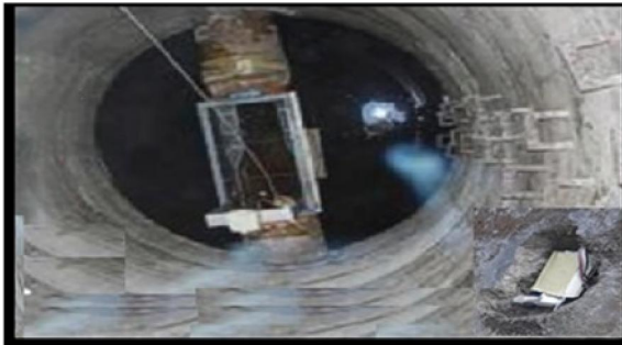
Fig 5. Position of sensor at smart drainage
