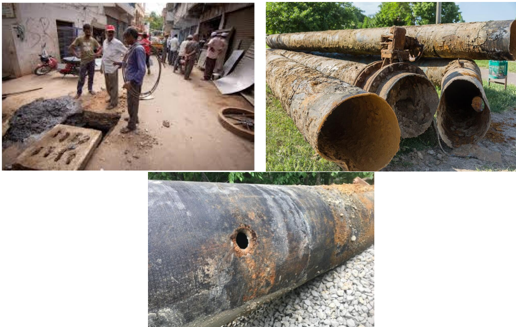
Fig. 2. (a, b&c) Manhole blockage, Corrosion in Industrial Pipelines & Crack in Pipes ( https://www.linkedin.com/pulse/challenge-getting-pipeline-failures-under-control-david-thompson )
