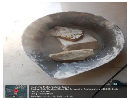
Preparation of Lime Slurry by Slaking of Lime Stone adding water into it
