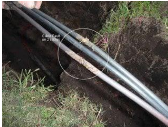
Figure 1: Underground cable fault
