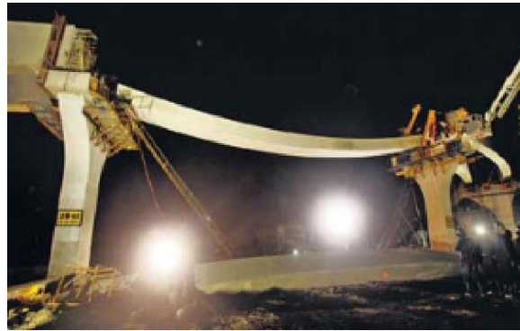
Fig.2 Elevated section of the tracks under construction came crashing down in Delhi Metro
