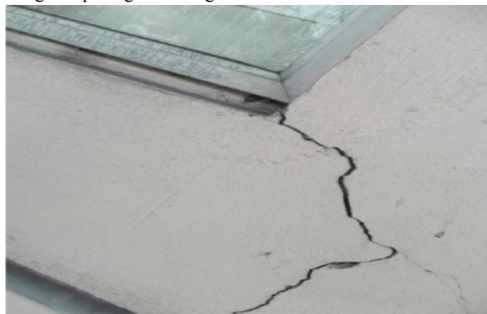
Fig 2 Vertical cracks at window sill level
