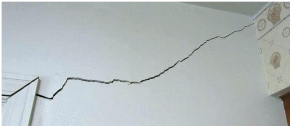
Fig.5.2 DIAGONAL CRACKS IN BRICK MASONRY WALL OVER LINTEL
