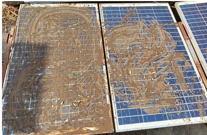
Fig. a Without Cleaning Solar Panel
