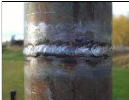
Figure 1. Corrosion in Welded Joints DOI: 10.48175/IJAR SCT-11906
