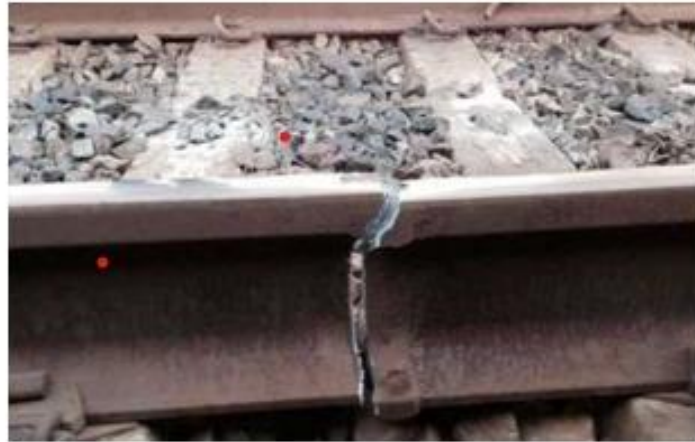
Fig. Cracks on Railway track
