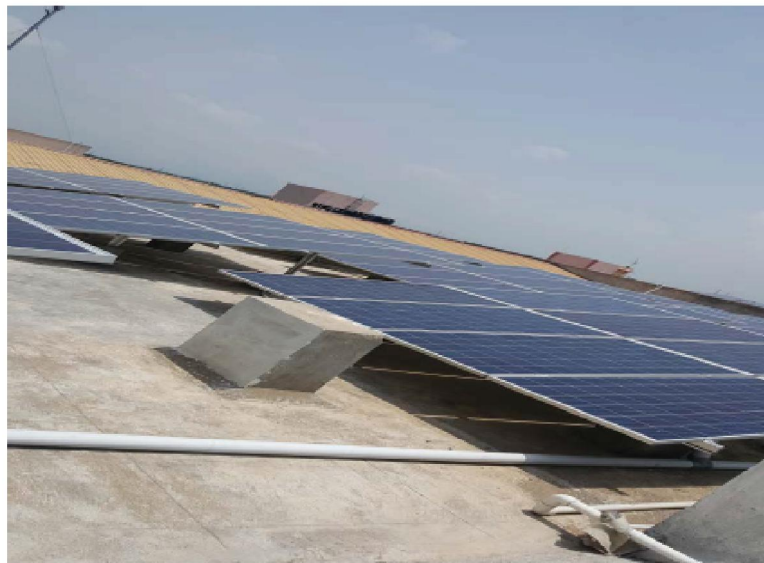
Figure 1.2: A Rooftop Installation of PV sheets.
