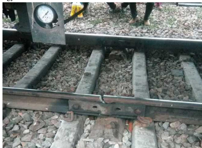
Fig: Crack on Railway Track DOI: 10.48175/568
