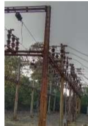
33kV Bus Structure
